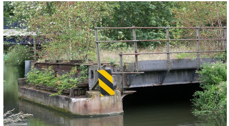
Fixed bridge span on the station side of the Swing Bridge showing the landing deck below the track level with the controlling capstan behind the yellow and black board. 2010
