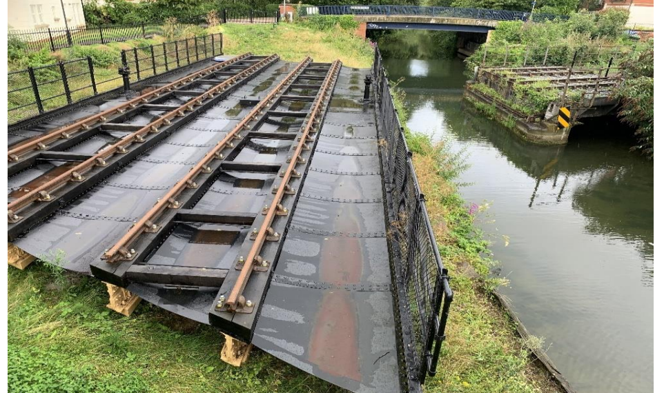
View of restoration work, including the new fixed span track, taken from passing train in August 2023
