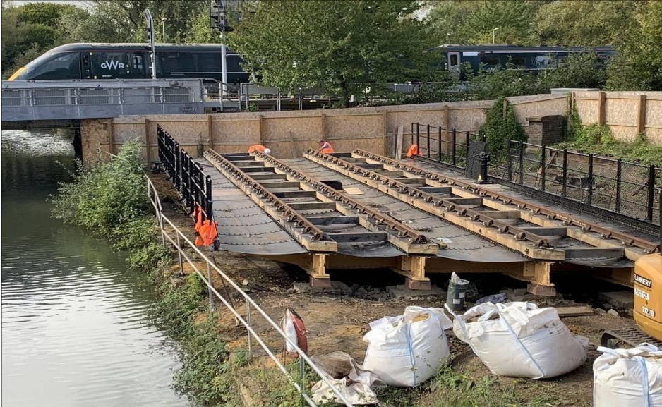
The Completed deck plating and track restored to original design above the original restored 1851 bridge beams and turning gears in 2022
