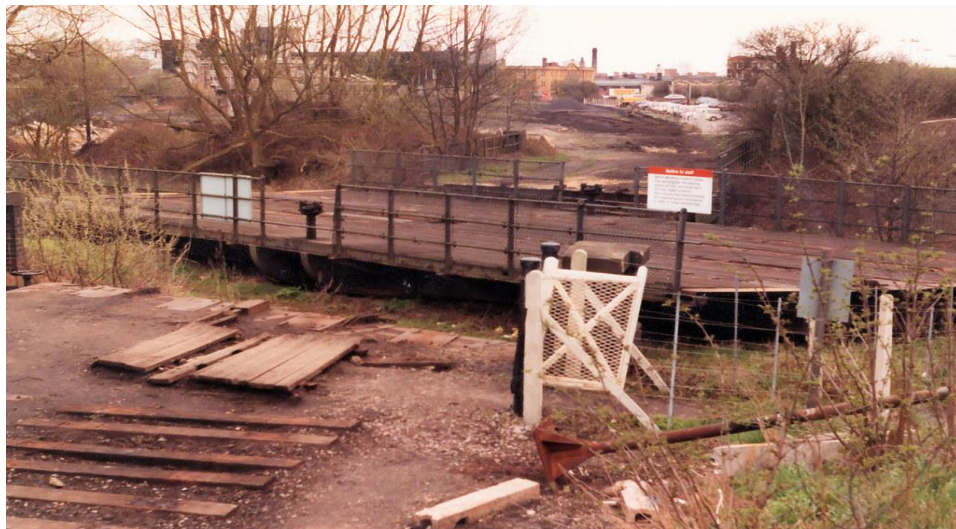
Bridge after removal of track and turned out of use in 1985 before LNWR track recovered from Bicester was placed on top and the gears wedged to stop unofficial use by building contractors until the restoration and transfer to the Oxford Preservation Trust in March 2021
